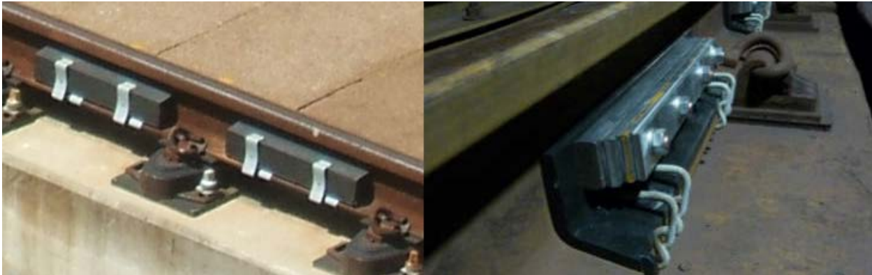
Figure 3 Installed rail damper examples
