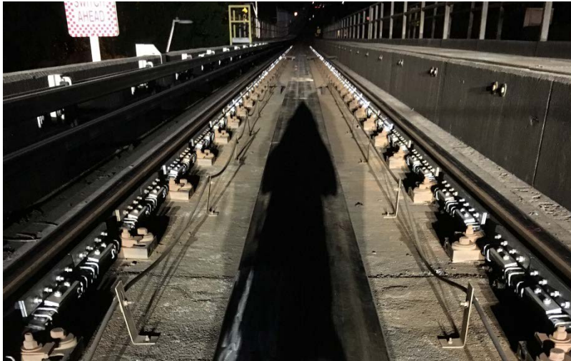
Figure 5 Nanaimo Outbound Track with Rail Dampers
